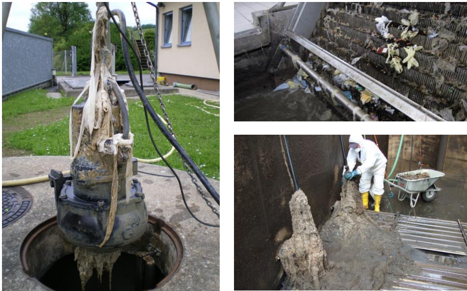
Figure 1: Wet wipe clogging in a rake system (top right), clogging pumps (left) and other treatment plant systems (bottom right).
