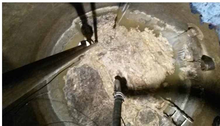
Figure 5: View from above of the floating layer of a pump station in Mürzzuschlag
