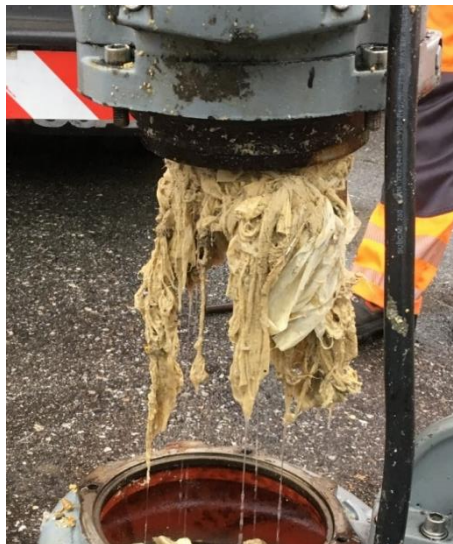
Figure 6: Disassembled pump with plug of wet wipes from a pump station in Kapfenberg
